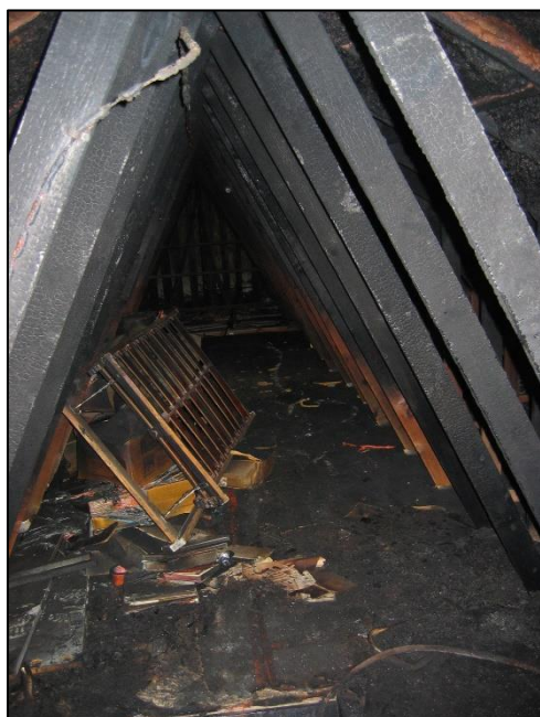
figure 2 View from the ladder into the attic. The photo shows how narrow the attic space is. (Photo: Fire service Westhoek – station Diksmuide)
