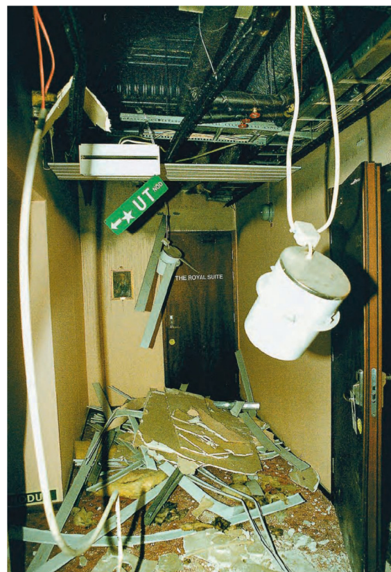
Fig 1.4 Consequences of a smoke explosion. (Photo: Roland Stregfelt, www.msb.se )
