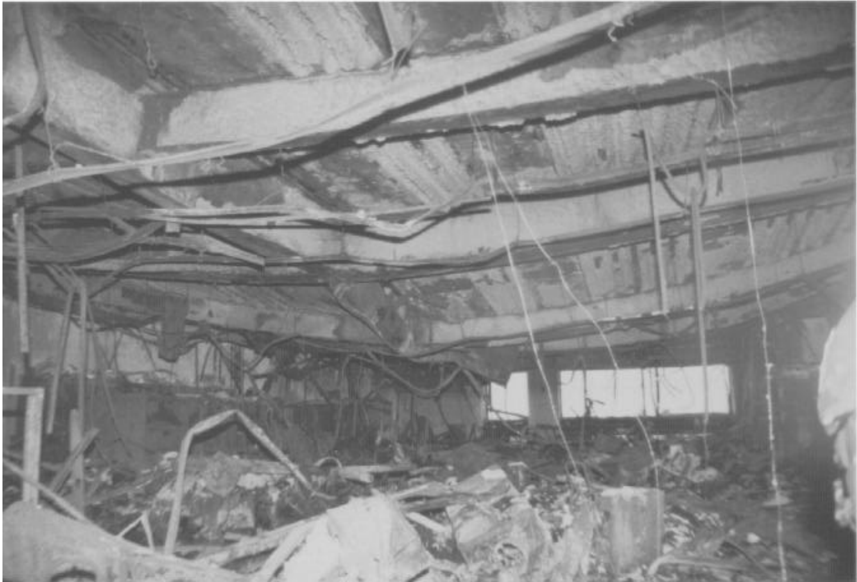
Here and in the next three photos are interior views of floor areas after the fire. Note the total consumption of the available fuel and sagging of the floor deck of up to three feet between columns.
