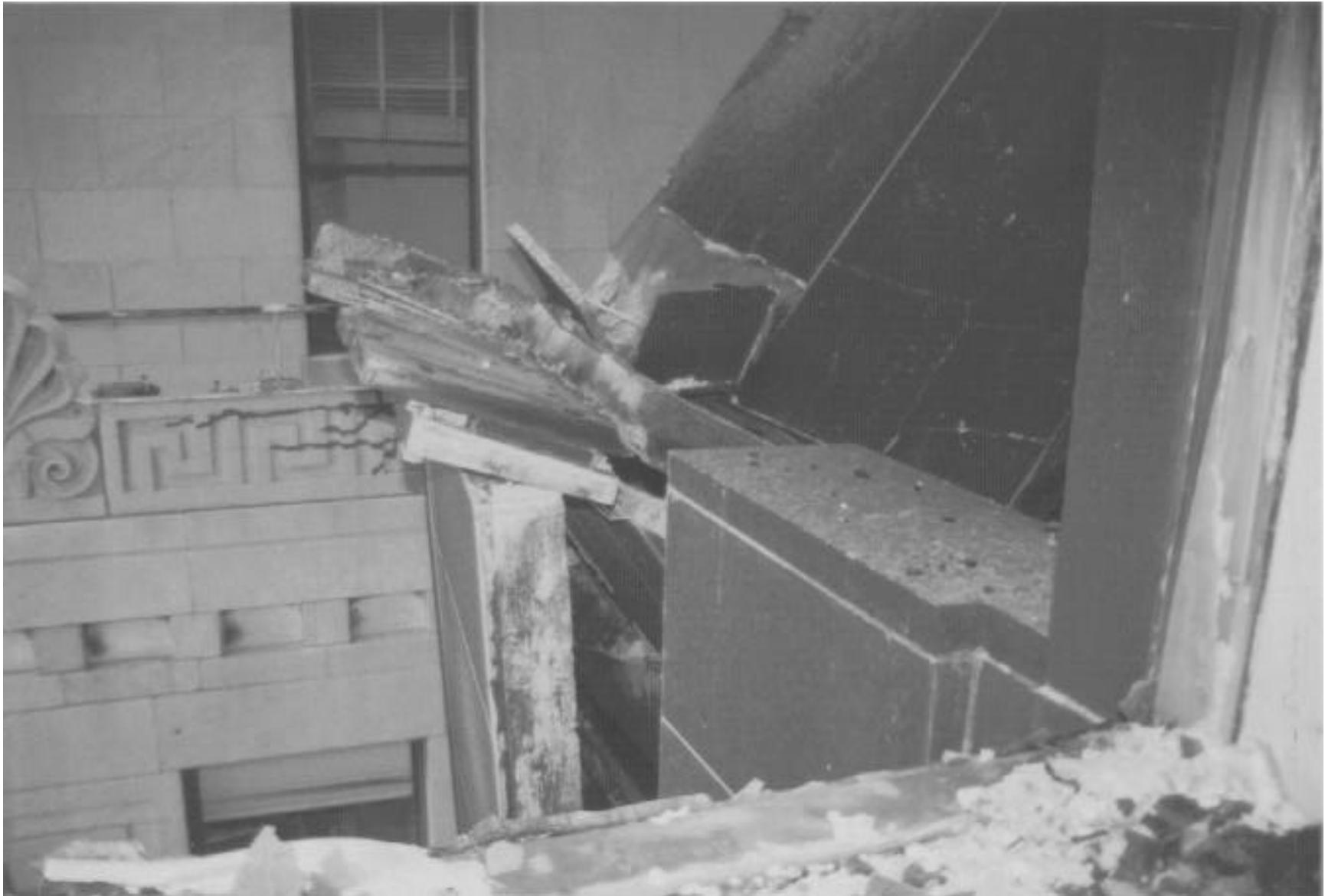
Here and in the next two photos exterior granite panels from the east stair tower were dislodged due to the thermal expansion of the steel frame of the building.
