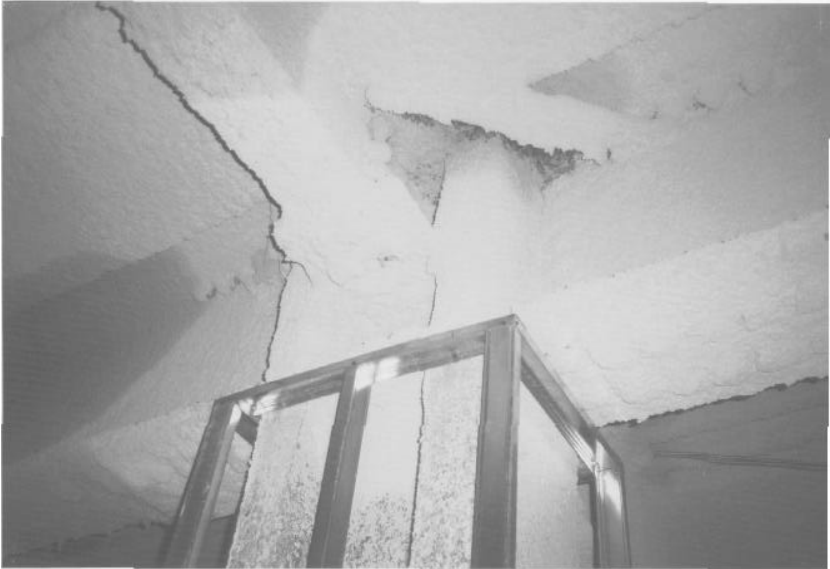
Detail of typical Type 1B construction, 6th floor. Note the spray-applied fireproofing and framing for gypsum wallboard.
