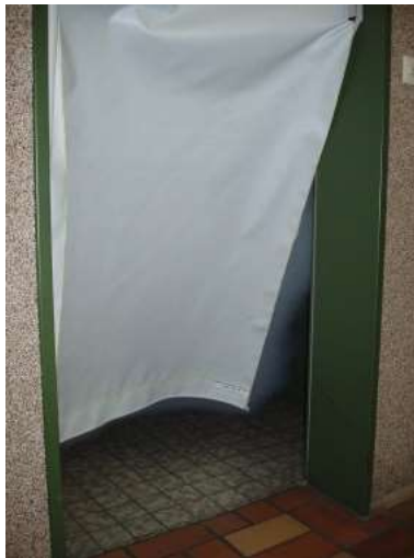
Figure 3: Influence on the characteristic of the fresh air flow into the fire compartment by a smoke blocking device with a curtain nearly covering the whole opening and forcing the fresh air flow to go in low
